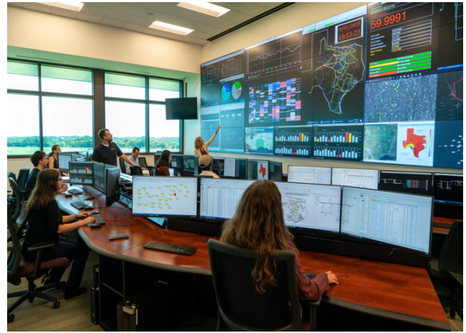
Fig. 8. Control Center Laboratory at Texas A&M University
