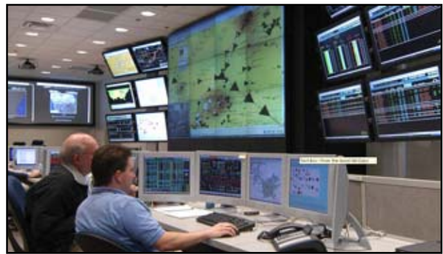
Figure 1: TVA Regional Operations Center (ROC), 2006
